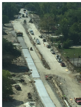
RIGHT: This aerial photo from ODOT was taken Sept. 18, showing the paving progress on East 105th Street between Cedar & Quincy Avenues.
